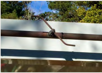
↑ 'Catherine wheel' sprinklers send water up onto the roof and down the walls to protect against fire.
