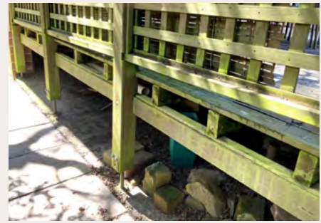
↑ This treated pine deck and screen would be vulnerable to ember attack during a fire. Enclosing the space underneath with a fire-resistant skirt would be a good start.
